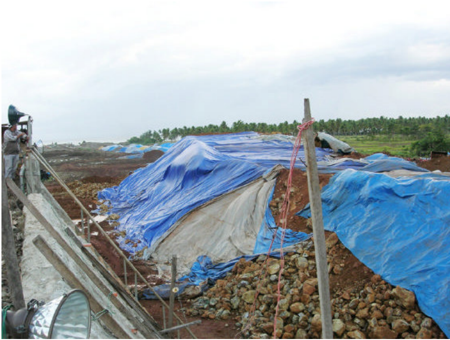
Figure 49: View of NNMDC Stockyard Looking South – Tarps Covering Material Ready for Shipment.
